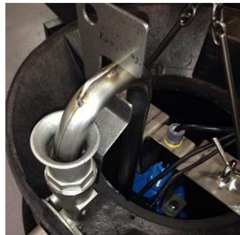
• Discharge Elbow “Seated”
